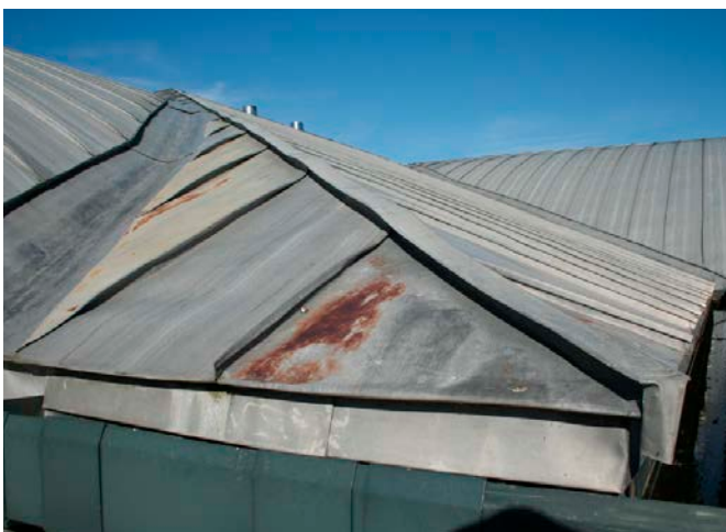
Figure 12: Discolouration of lead-rich terne-coated stainless steel
